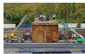
Concrete may be poured for the center pier of the Grant Street Bridge by the end of next week.
