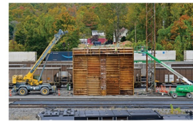
Concrete may be poured for the center pier of the Grant Street Bridge by the end of next week. Staff photo by Jessica Nuzzo
